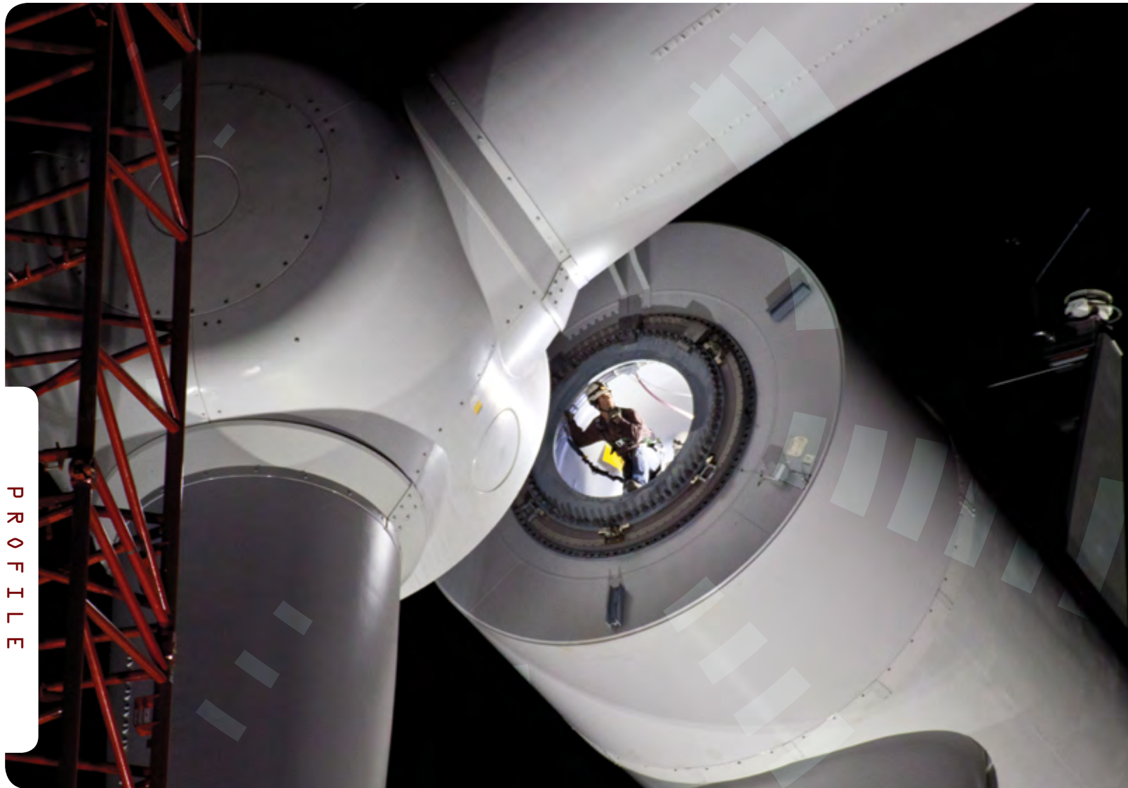
ON THE COVER AND ABOVE: A SIEMENS WIND TURBINE TECHNICIAN LEANS OUT THE NACELLE HATCH ATOP A NORTH DAKOTA WIND TOWER AS A ROTOR IS HOISTED INTO POSITION LAST DECEMBER. CONTRACTORS AND MINNESOTA POWER PERSONNEL ELECTED TO “FLY” SOME OF THE ROTORS BY CRANE DURING NIGHTTIME HOURS LAST WINTER BECAUSE NORTH DAKOTA WINDS ARE USUALLY CALMER AT NIGHT. WORK PROCEEDED UNDER FLOODLIGHTS DURING A NINE-DAY CONSTRUCTION PERIOD WHEN WIND CHILLS AT TIMES DROPPED TO 40 BELOW ZERO.
